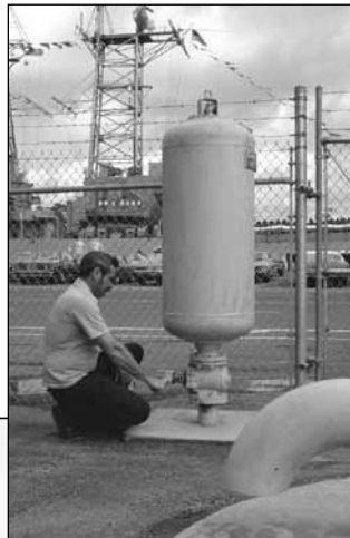
Refineries — Shock from pump starting and stopping
